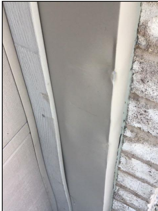
Mechanical damage noted around the garage...
