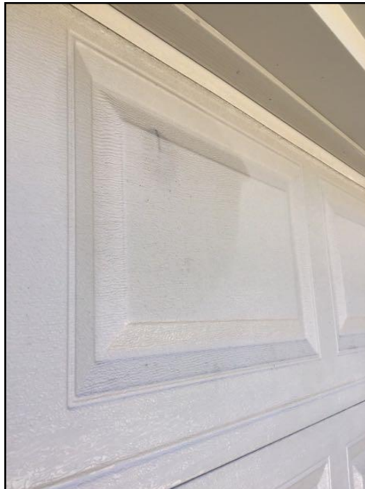
Minor mechanical damage noted on the garag...
