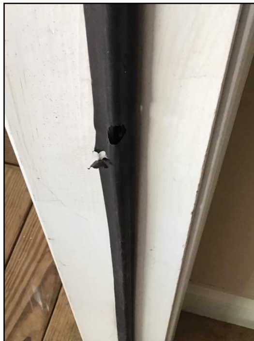
Damaged weather seal.
