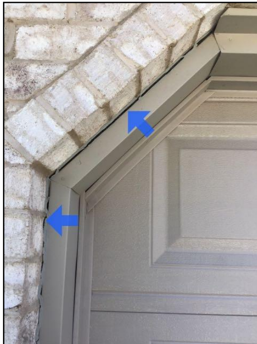
Recommend caulking around the garage door...
