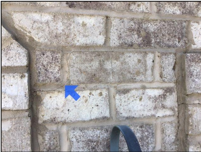
Minor cracks noted in areas. Repair/seal as...
