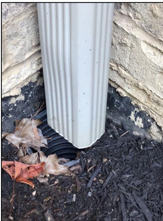
Gap between connection.
