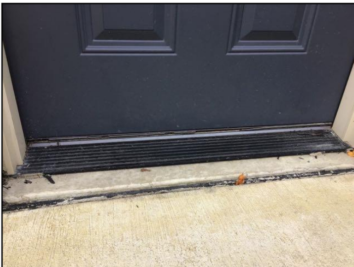
Damaged weather seal.
