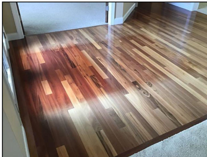
Ghosting noted on the floor. Repair area as...
