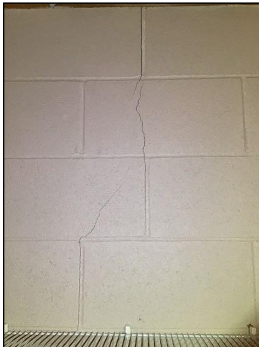
Crack(s) noted on the basement foundation....
